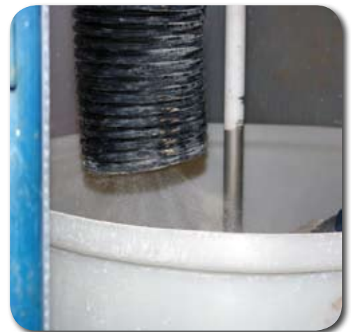
Local exhaust ventilation controlling fugitive emissions during precursor mixing at a primary nanoscale metal oxide production facility.
