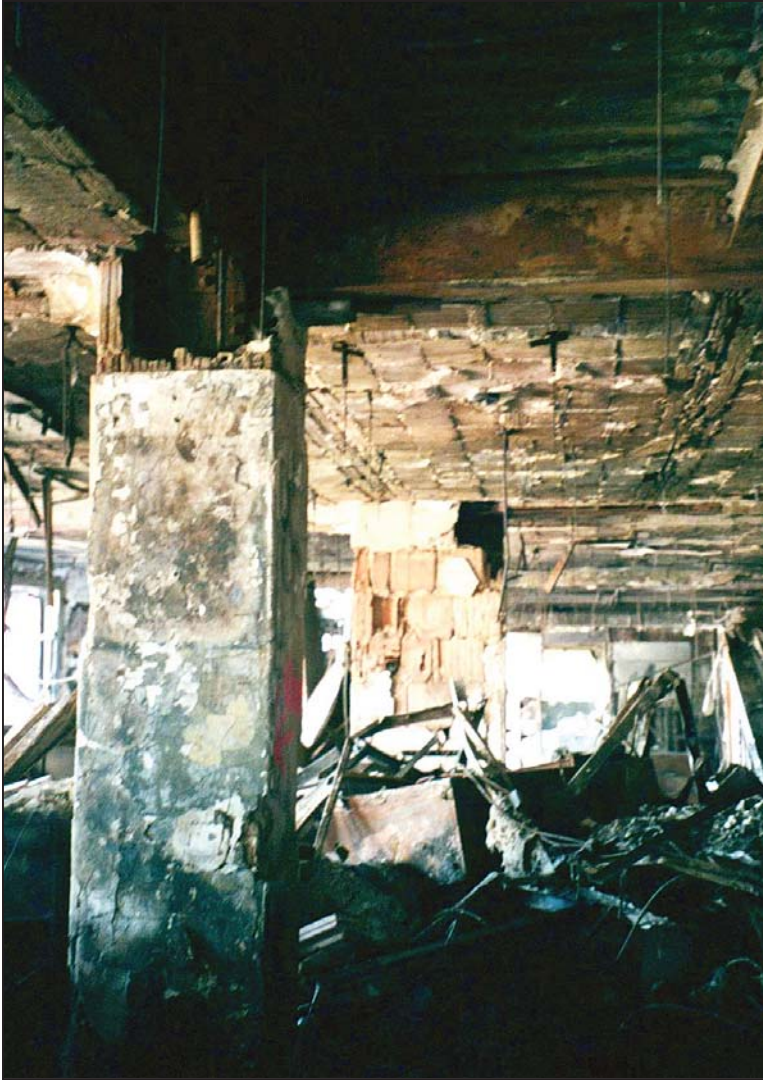
Figure 7-16 Buckling damage at top of column on floor 8 of 90 West Street. Note the loss of fire protection at the top of the column.
