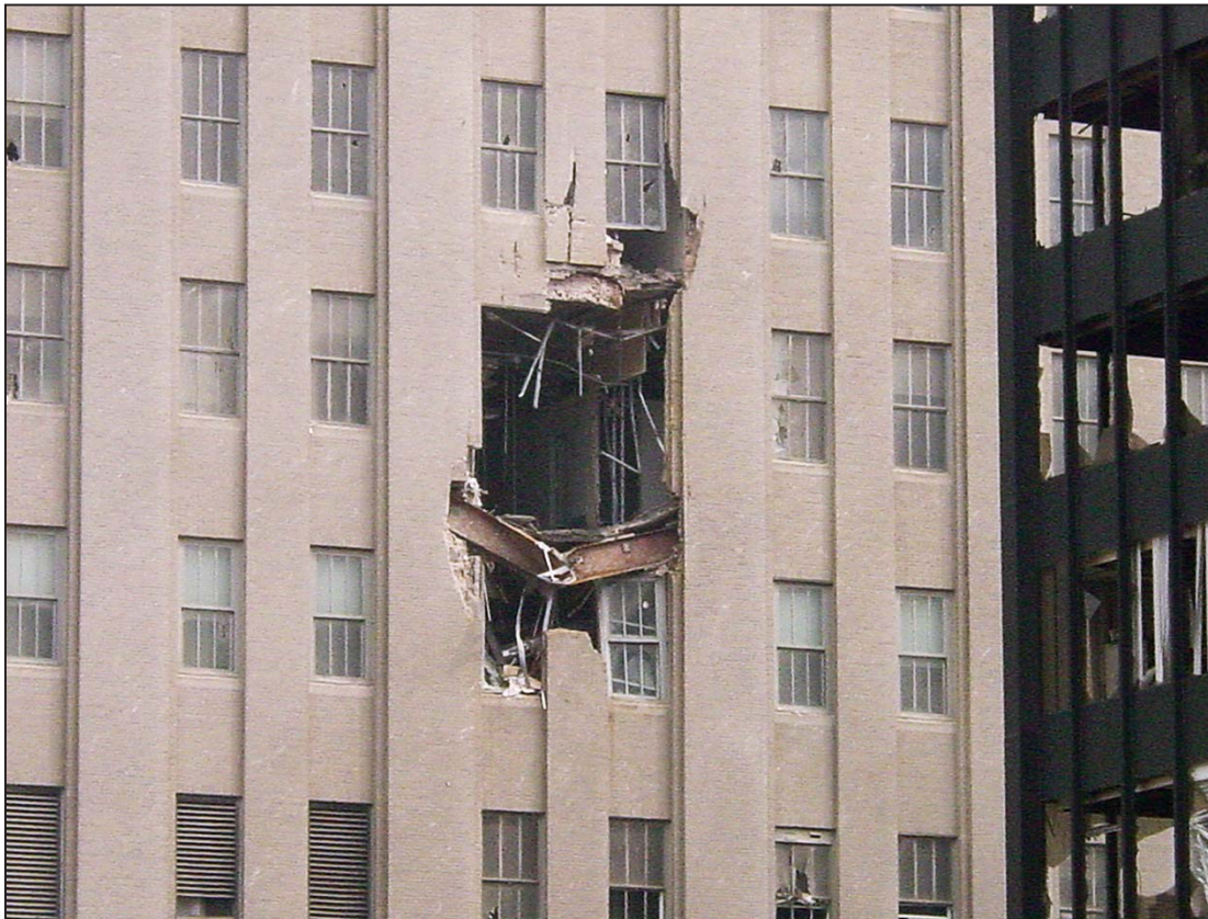
Figure 7-11 Verizon building – localized damage to south elevation (Vesey Street).
