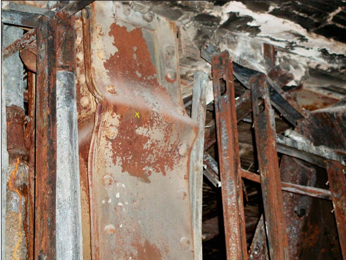
Figure 7-17 Buckling damage at top of column on floor 23 of 90 West Street.
