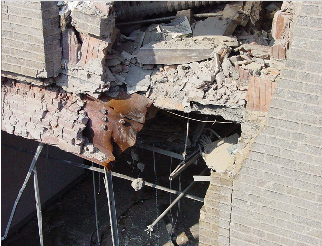
Figure 7-12 Verizon building – detail of damage to south elevation (Vesey Street).
