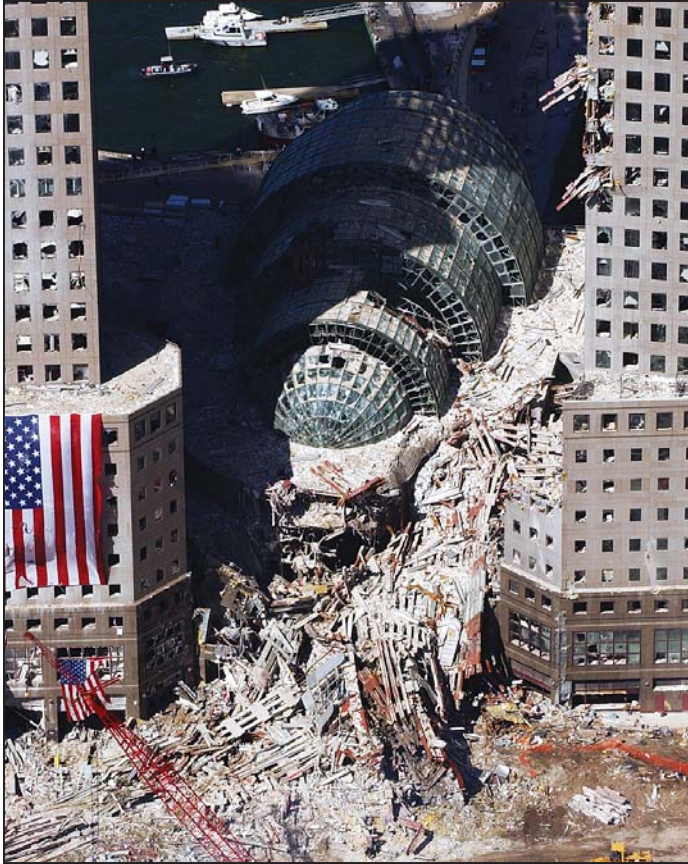
Figure 7-3 View of Winter Garden damage from West Street, with WTC 1 debris in front of WFC 2.
