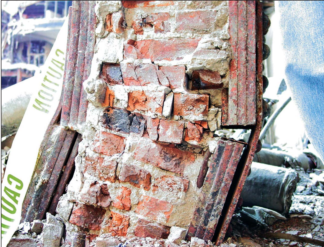
Figure 7-9 Verizon building – column damage on east elevation (Washington Street).
