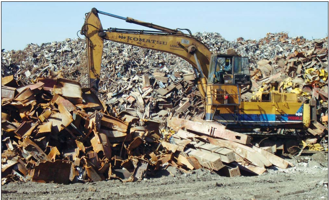
Figure D-3 Pile of unsorted, mixed steel (background) with sorted, large steel pieces (center) being lifted and cut into smaller pieces (left).
