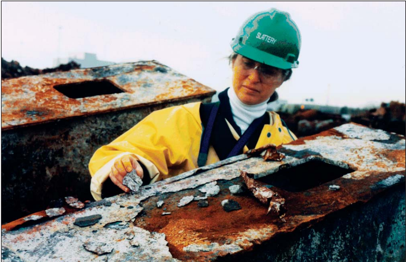
Figure D-16 Engineer inspecting fire damage of perimeter column tree from WTC 1 or WTC 2.
