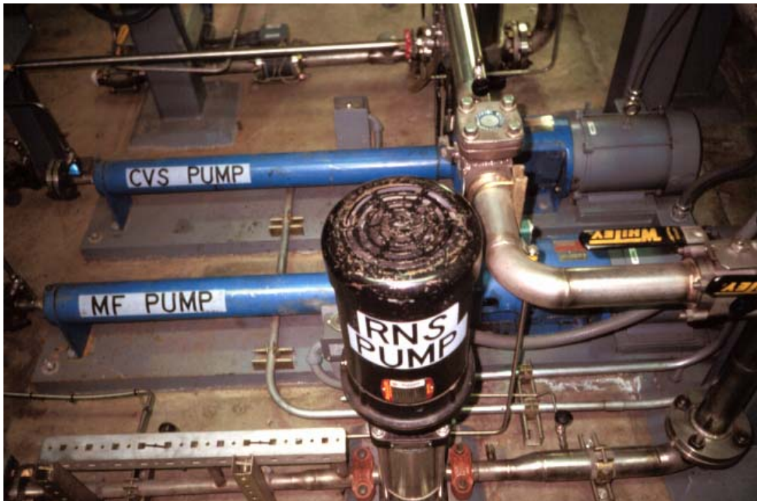
Figure 3.26. Image of RNS, CVS, and MF Pumps
