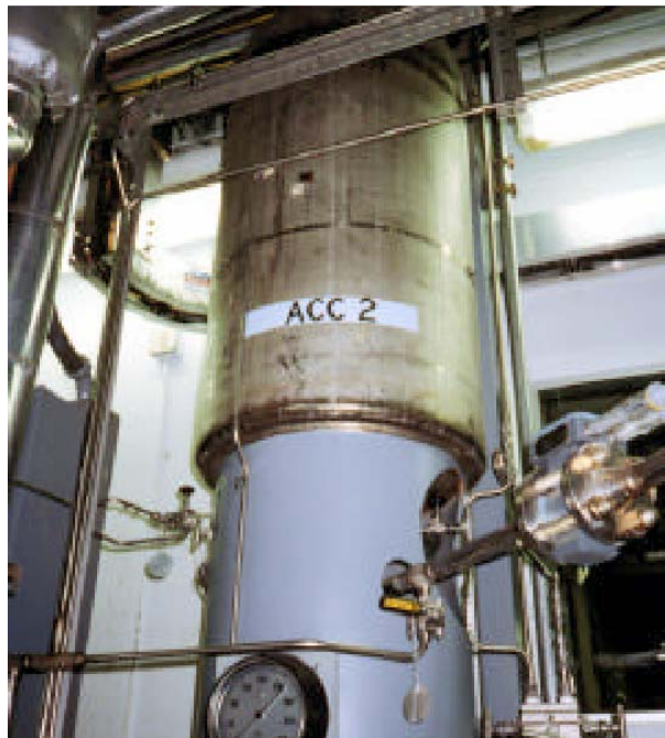
Figure 3.18. Photograph of One of the APEX Accumulators
