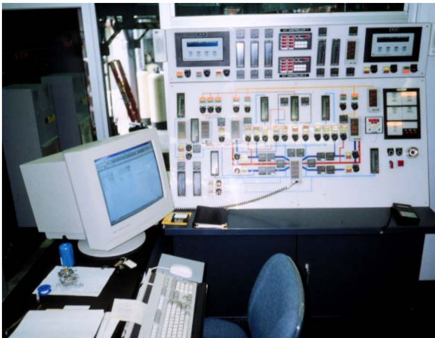
Figure 3.21. Photograph of the APEX Control Panel
