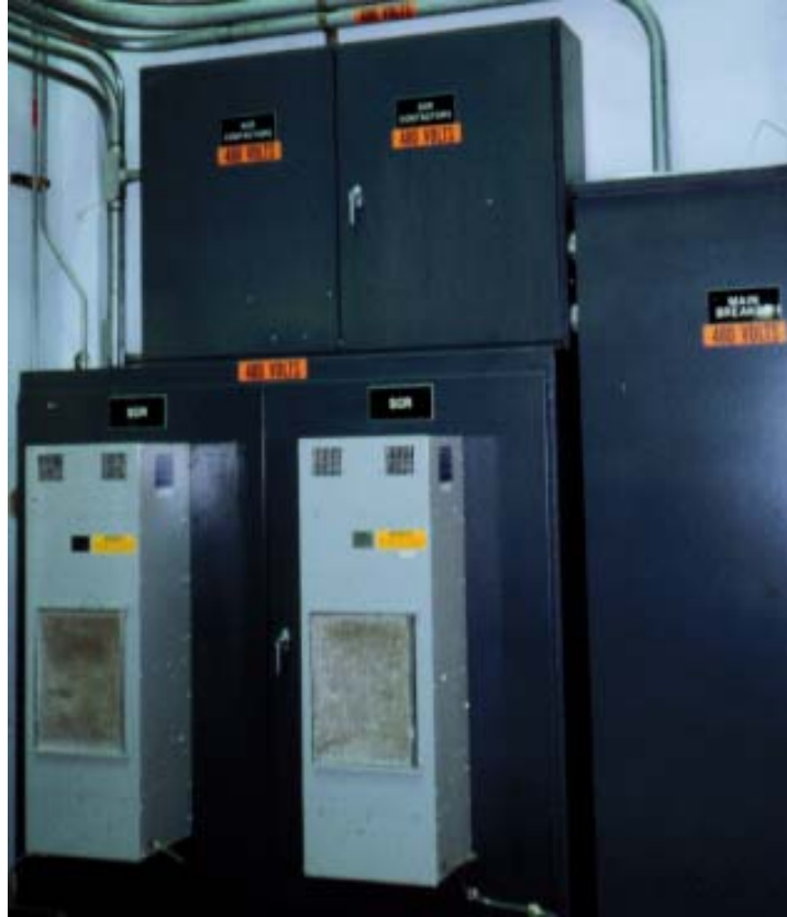
Figure 3.22. Photograph of the SCR Cabinet
