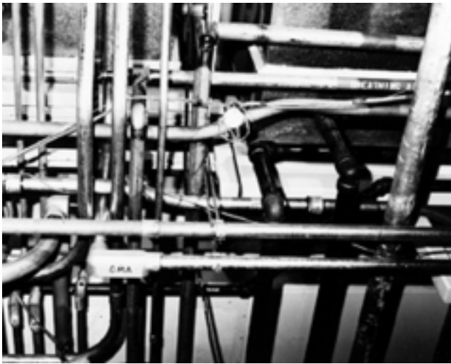
Piping in Building 371
