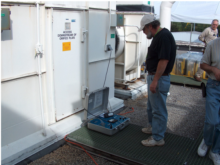
HEPA Filter Efficiency Testing
