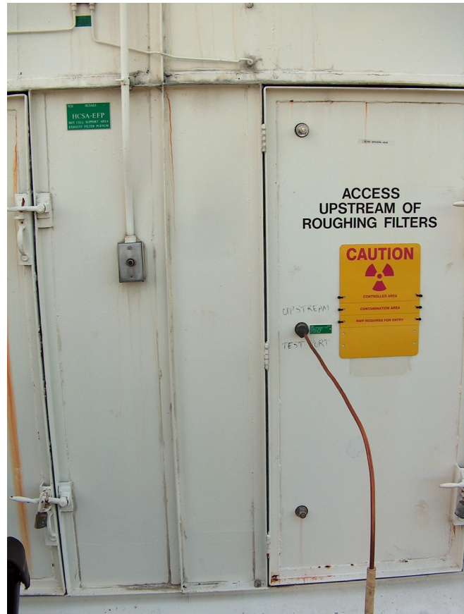
Hot Cell Support Area Exhaust Filter Plenum
