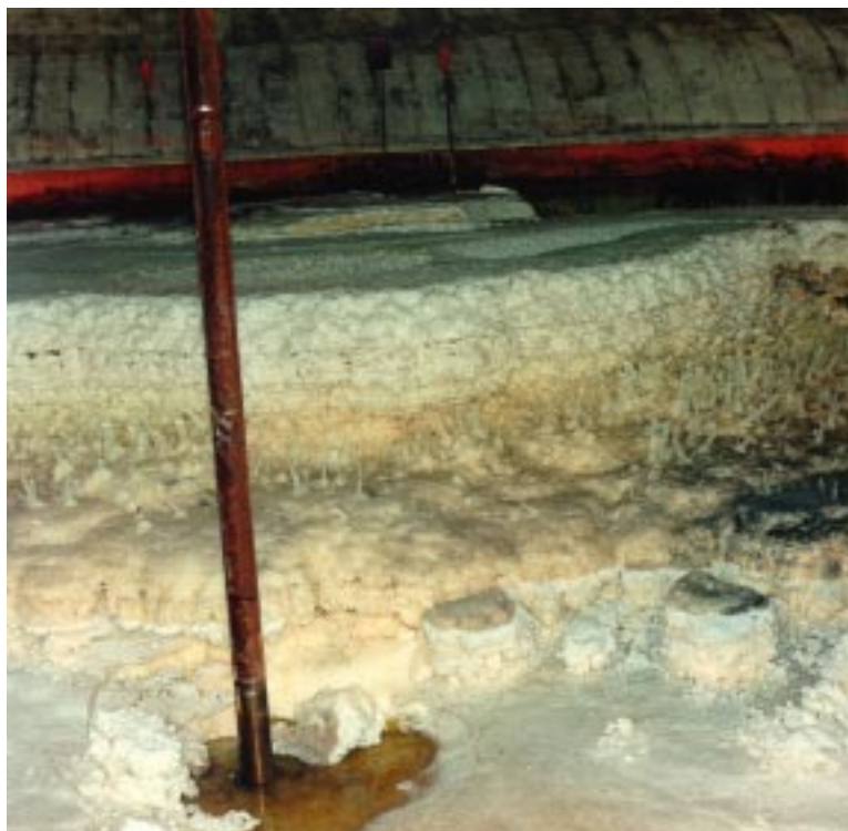
Inside a Tank in B Farm
