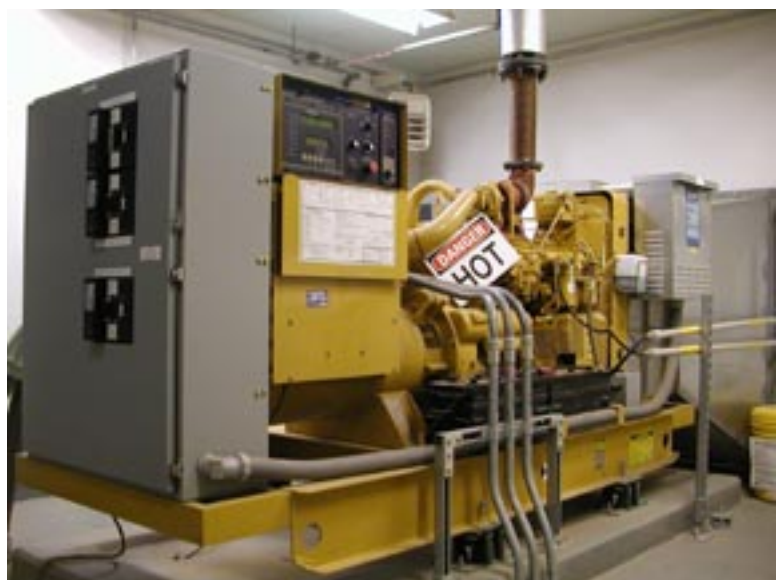
Aging Waste Facility Backup Diesel Generator
