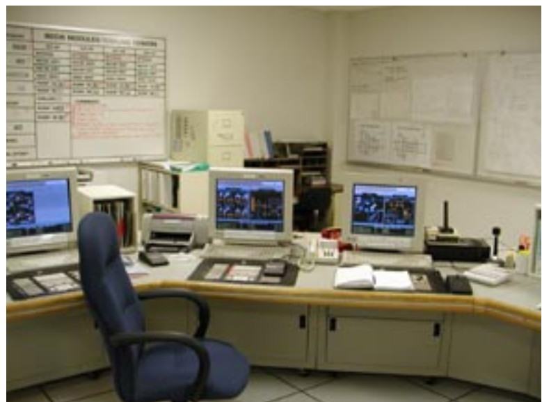
Monitoring & Control Station
