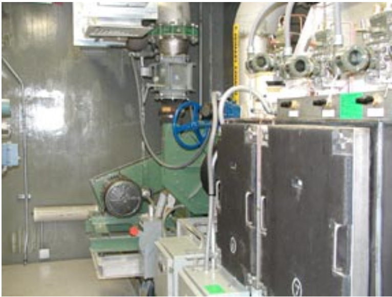
Primary Ventilation Fan in Background; HEPA Filter Train in Foreground
