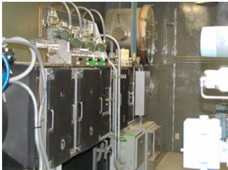
Primary Ventilation System HEPA Filter Train
