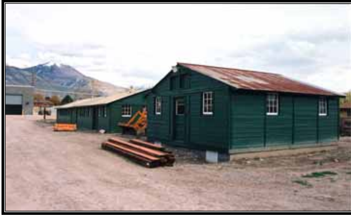
Figure 3.73 Pleasant Grove CCC buildings following partial rehabilitation. (Source: Barbara Boyer, Bureau of Reclamation)
