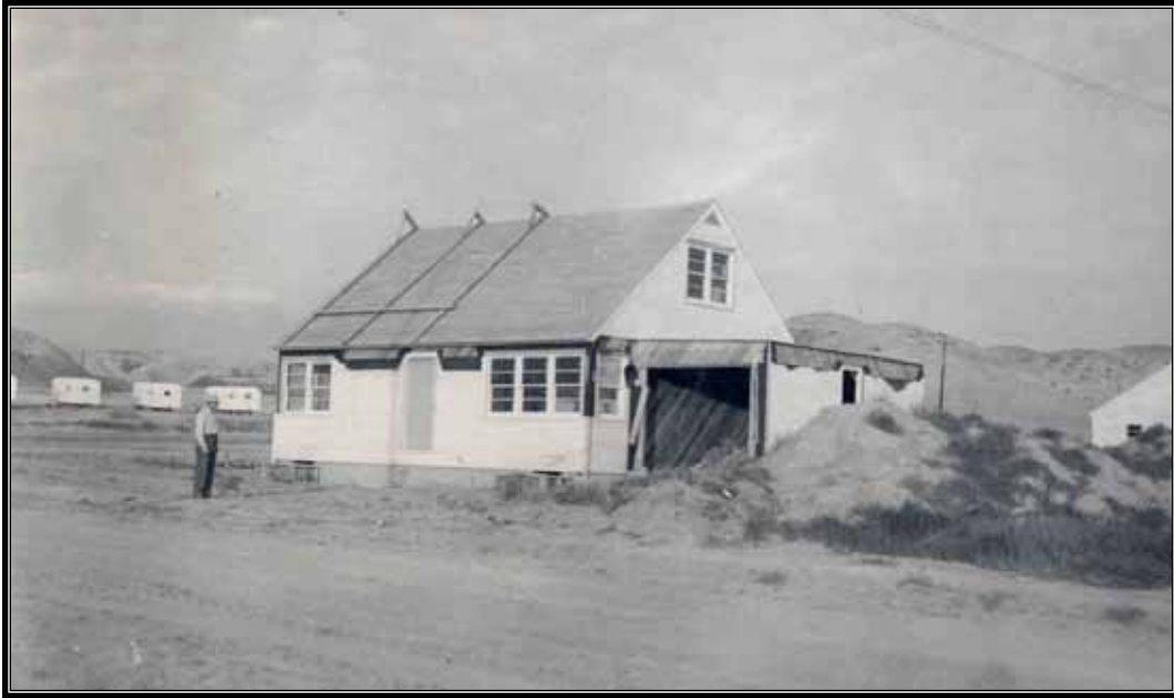
Figure 4.19 Missouri River Basin Project, Tiber Dam government camp, Lower Marias Unit, Montana. One of the two five-room permanent houses under construction. The temporary two- and three-bedroom houses were similar but smaller and lacked attached garages. Photo taken September 12, 1952.
