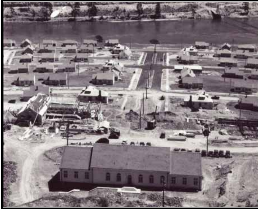
Figure 3.31 At bottom of photograph is a rear view of the administration building in 1935, still under construction.
