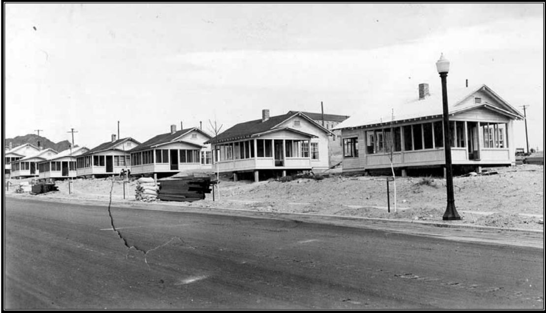
Figure 3.18 Identical three- and four-room temporary houses being built on Utah Street in April 1932.
