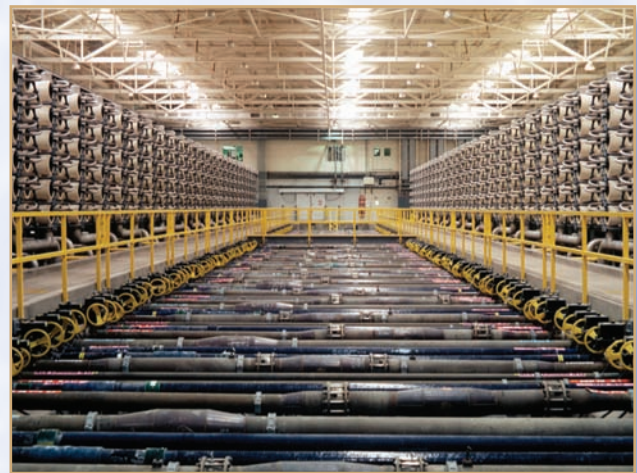
Yuma Desalting Plant
