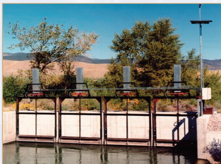
This four-gate diversion structure was retrofitted with an automation system that is solar-powered.
