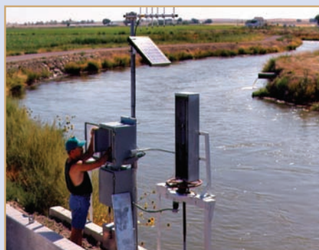
Solar-powered automated headgate
