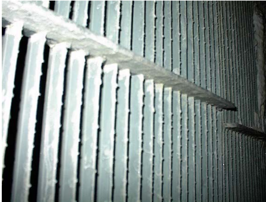
Figure 12.—Mist eliminators in the cooling jackets.
