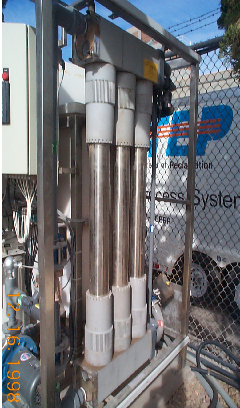
Figure 4.5.—Three Module Bank on Memcor Unit
