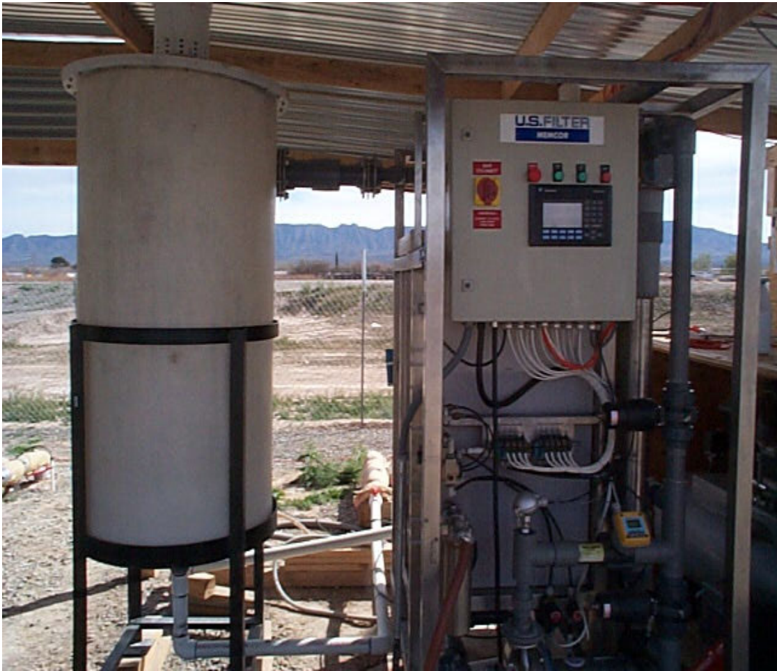
Figure 4.4.—Memcor Unit with Backwash Tank
