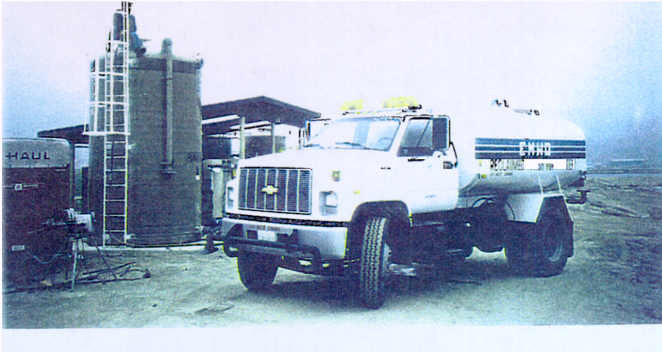
Figure 4.5.—Well water being pumped into the 5,000.gallon RO feed tank.
