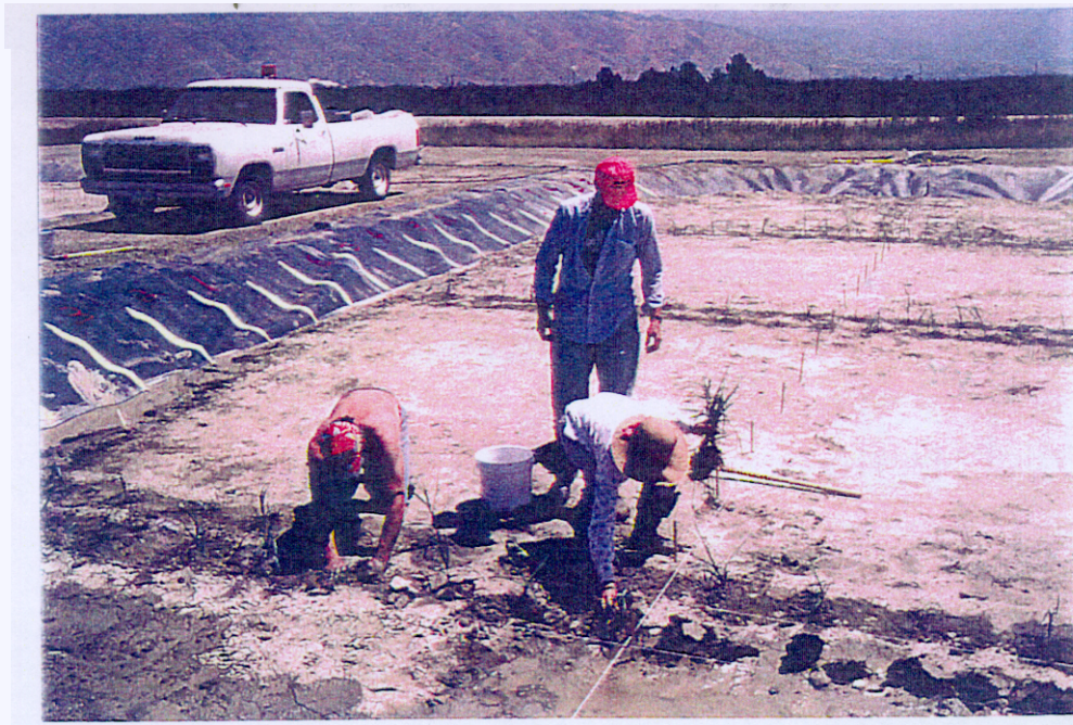
Figure 5.5.—Salt-tolerant wetland plants being planted on 45.7-cm (18-inch) centers in 3-foot-wide horizontal bands (refer to figure 5.4 for planting scheme).
