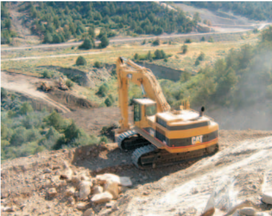
Excavation of Ridges Basin Dam, Colorado/New Mexico, viewed from top of right abutment.
