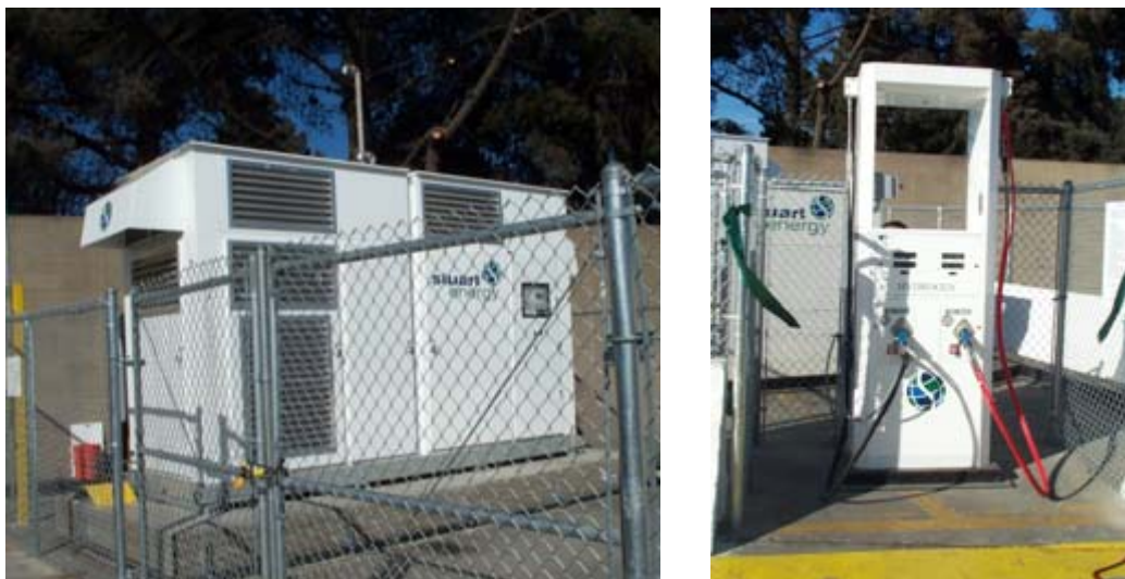
Figure 4. Electrolyzer (left) and dispenser (right) at Richmond Division
