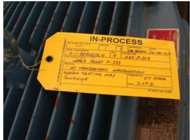
A test tag on equipment being transferred to operations
