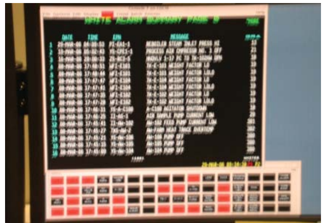
A computerized status board with red indicators for alarms
