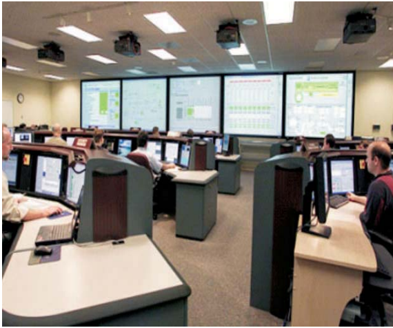
Facility Operations Control Room
