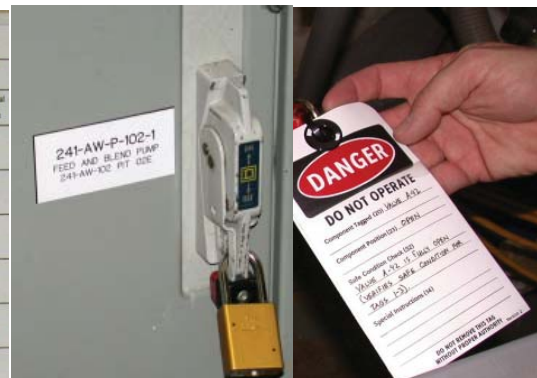
A lockout/tagout logbook, lockout on a circuit breaker, and tagout on a valve
