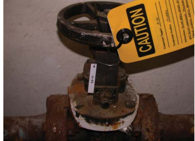
Shift supervisor's caution tag on a valve, which provides special instructions
