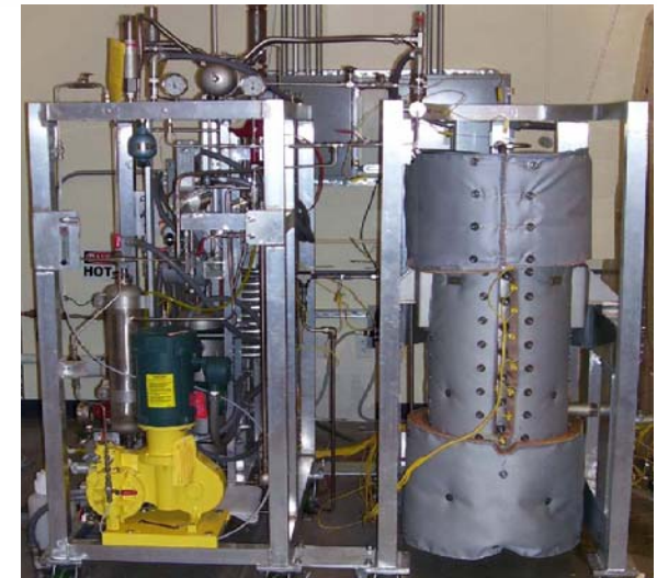
10 kg/day Hydrogen Pilot Plant
