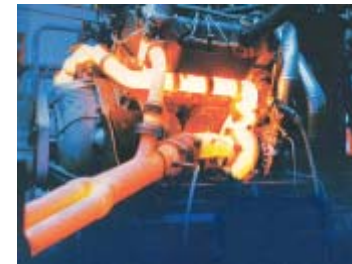
Exhaust System Waste Heat
