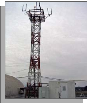
A 1-kW fuel cell system has been providing power for this FAA radio tower near Chicago for more than three years. (Photo courtesy of ReliOn)
