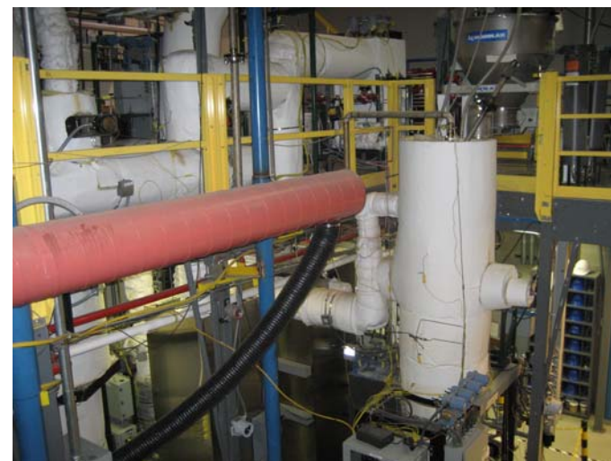
NREL 3 kg H 2 /hour Biomass Gasifier
