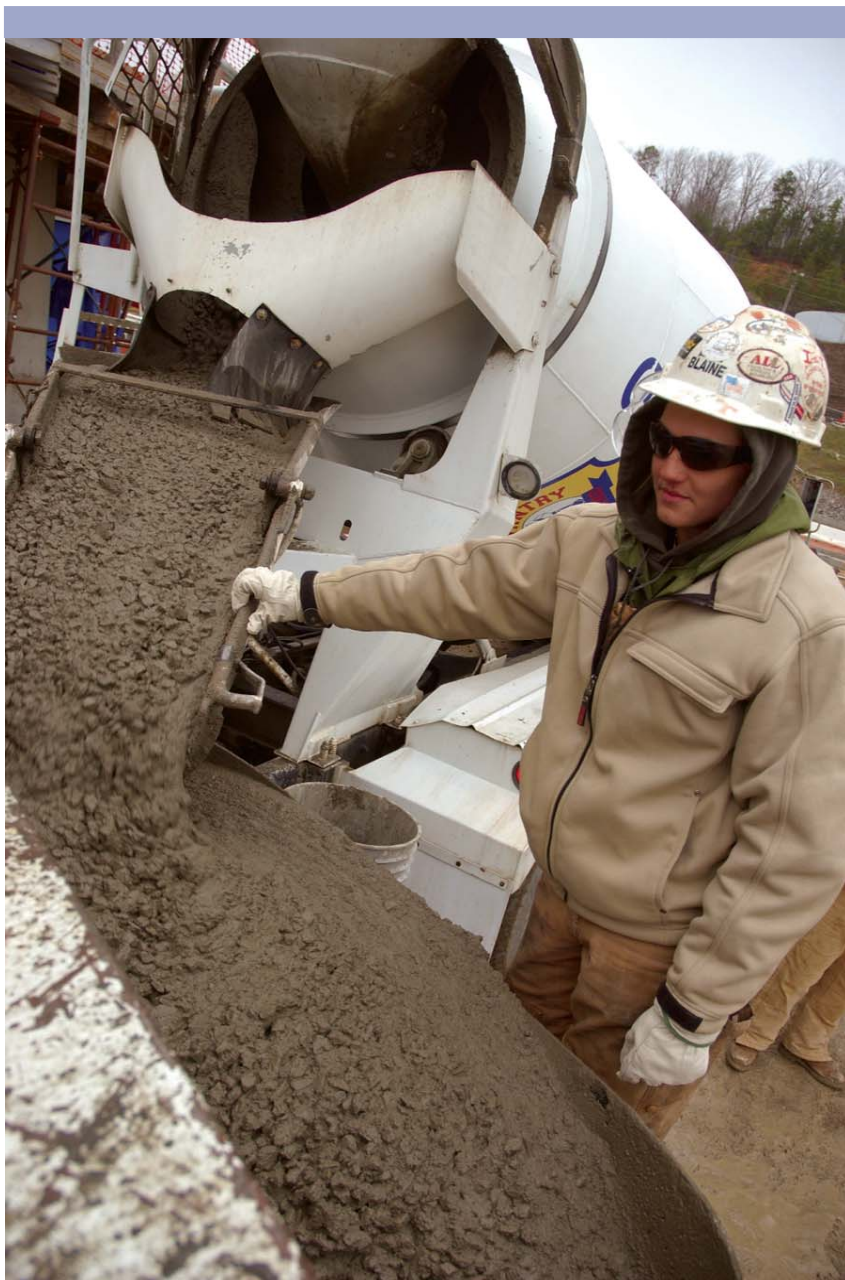
SITE MODERNIZATION: Concrete from a mixer truck is emptied onto the conveyor of a concrete pump direct to the roof of the Highly Enriched Uranium Materials Facility.
