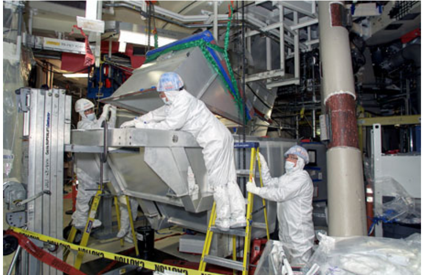
NIF: Workers install beampath onto a mirror frame under the target chamber.
