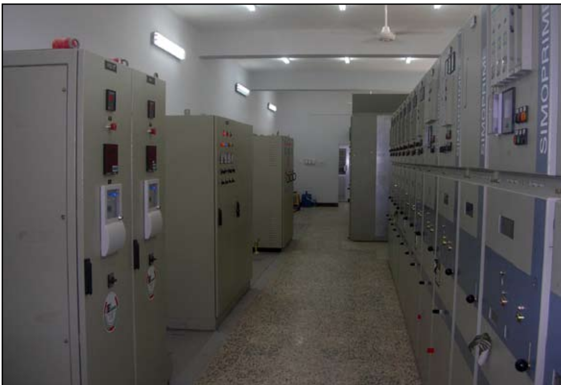
The control room at Maysan Plastic 33/11 kV substation project will ensure stable electrical supply within the Maysan province and supply more electricity to the people of Maysan.
