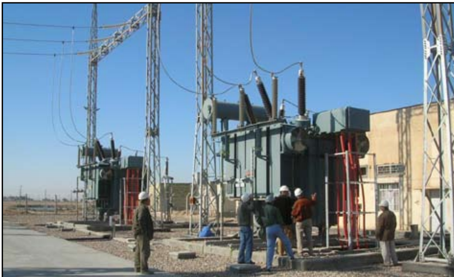
Engineers check work accomplished on two 63 megavolt amps transformers at cluster pump station one, North Rumaylah, Basrah.
