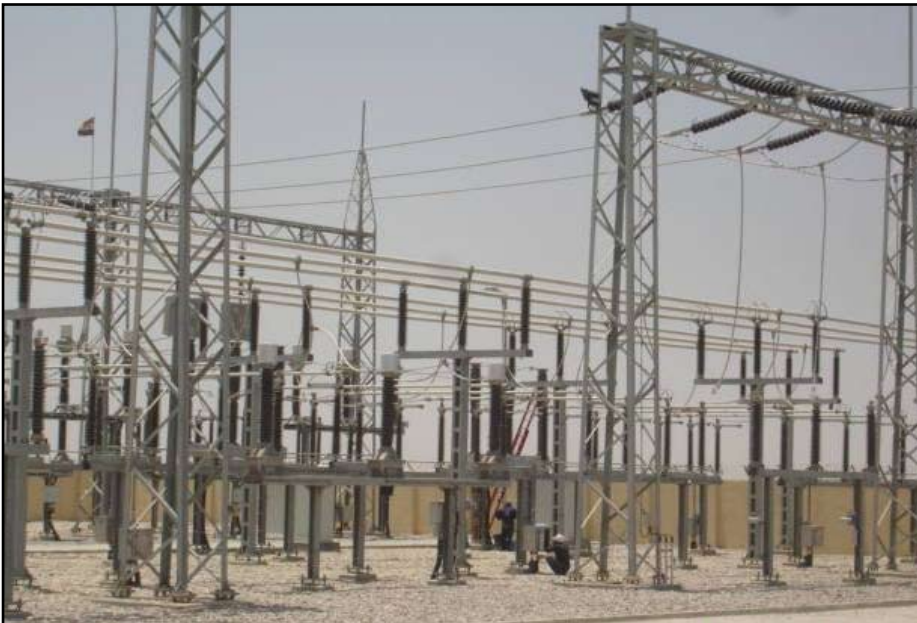
Left: Al-Garma 132kV substation project will serve more than 13,000 residents north of Basrah city.
