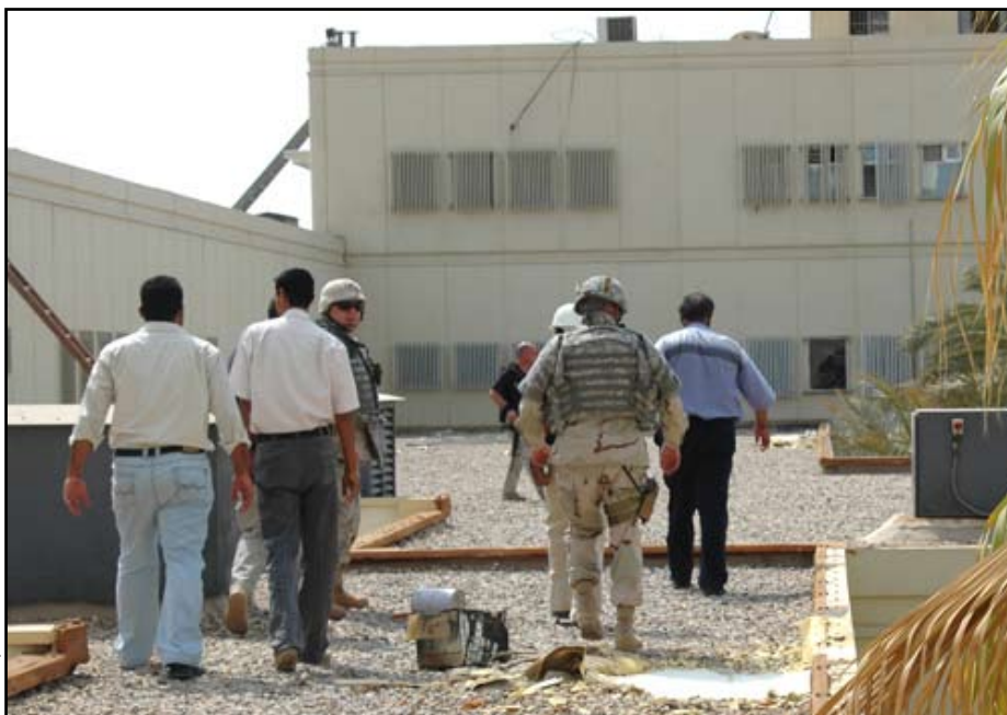
U.S. Army Corps of Engineers and construction contractors look over roof work to be completed on renovation of the hospital.
