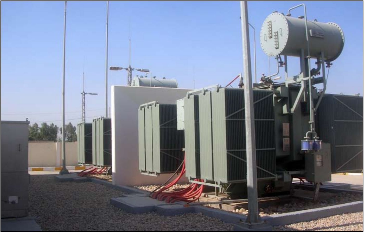
The two, 31-megavolt transformers will upgrade the area's electrical distribution benefiting more than 785,000 residents.
