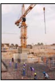
A crane operator lowers rebar to workers preparing the foundation of the Al Mamoon Telecommunications Center.
