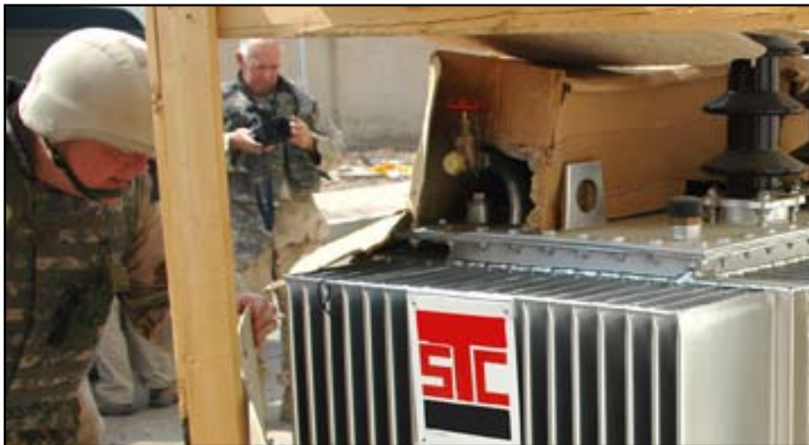
Resident Engineer John Overfield looks at a transformer remaining to be installed as the contractor finishes work on the Nasiriyah Maternity and Pediatric Hospital. John Connor, public affairs officer, videotapes the visit.
