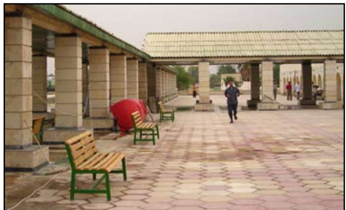
Renovation of walkways, platforms and the existing station buildings bring the Basrah station into usable condition. (USACE photos by A. Al Bahrani)
