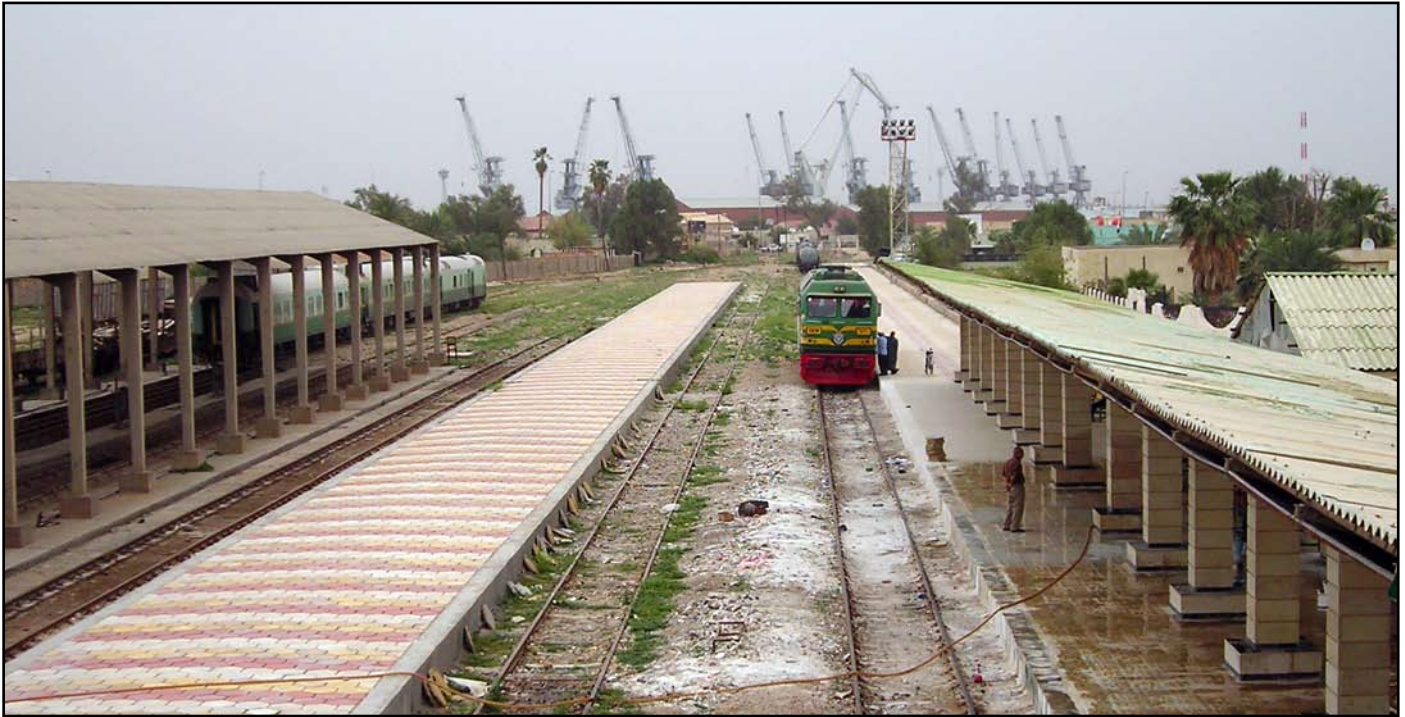
Workers wash down finished tile work on the Basrah platform as renovation work is completed on the $480,000 project.
