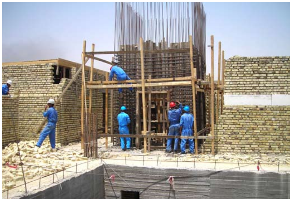
Workers on the second floor tie in rebar before concrete placement for an elevator shaft.
