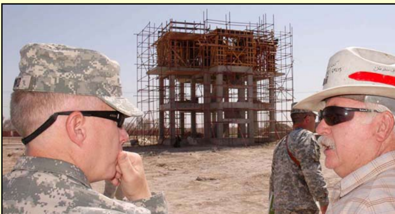
Project Engineer Andy May, right, who has been with USACE for more than four years in Iraq, shows Brig. Gen. Jeffrey Dorko the Taji Training Facility 9-meter-high rappelling and fast-roping tower which will be used by Iraqi army soldiers. (USACE photo by Norris Jones)
