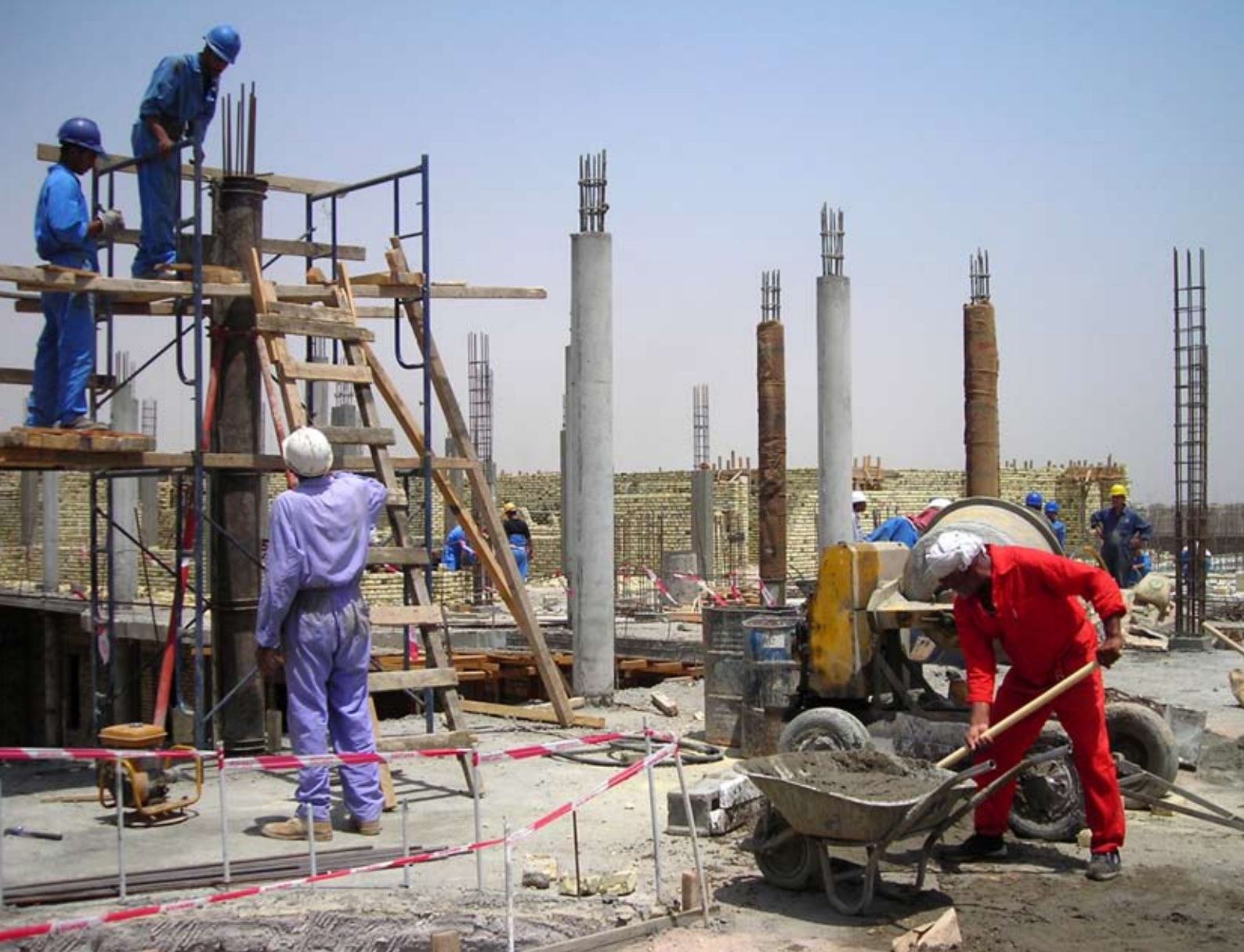
Iraqi workers mix concrete to place roof supports at the Basrah Regional Courthouse in Al Basrah Province. The $10 million courthouse scheduled to open by the beginning of 2008. The project currently provides more than 300 Iraqis with jobs in the area and has been a boon to the local economy. (USACE photos by Alaa Al Bahrani)
