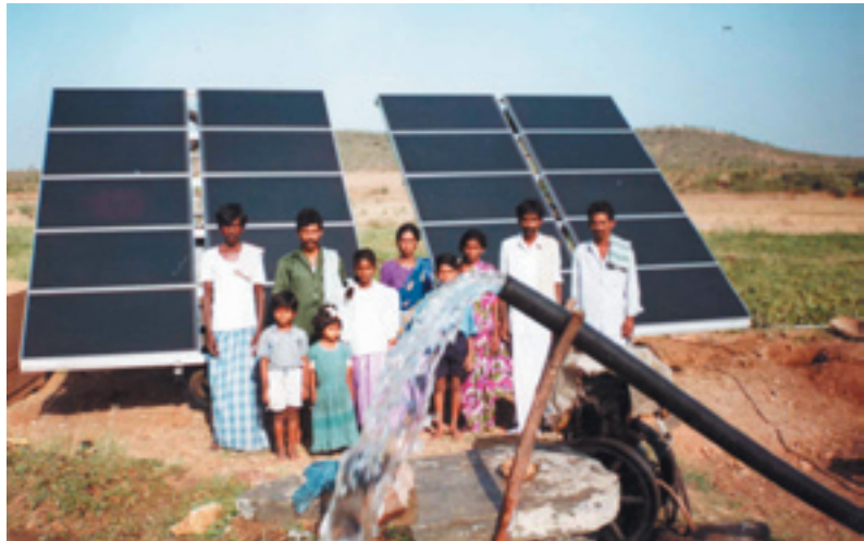
Solar powered pump in India installed as part of an Indian Renewable Energy Development Agency project.
