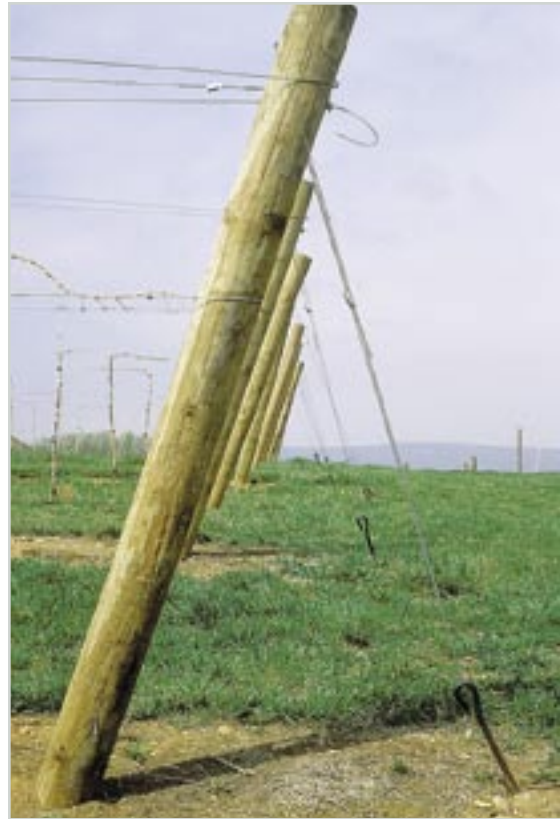
FIGURE 23. End posts are set 3 feet in the ground at a 60-degree angle and anchored with a screw-type steel anchor.
