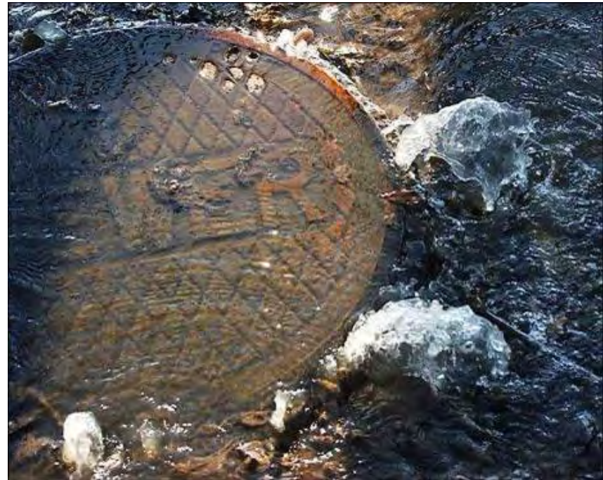
Raw sewage bubbles up from a man-hole cover along U.S. Highway 90 in Gulfport.
