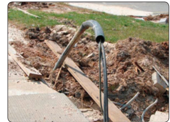
This is an example of damaged and exposed power lines and cables.
