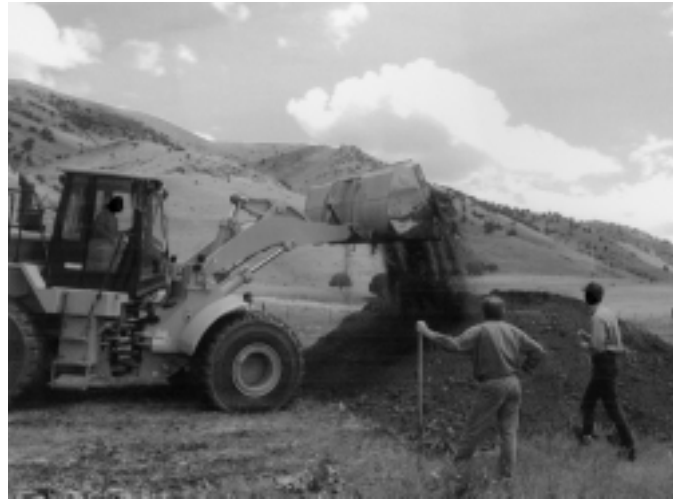
OIG employees assisting in excavation of APHIS site where homicide evidence was found. OIG photo.
