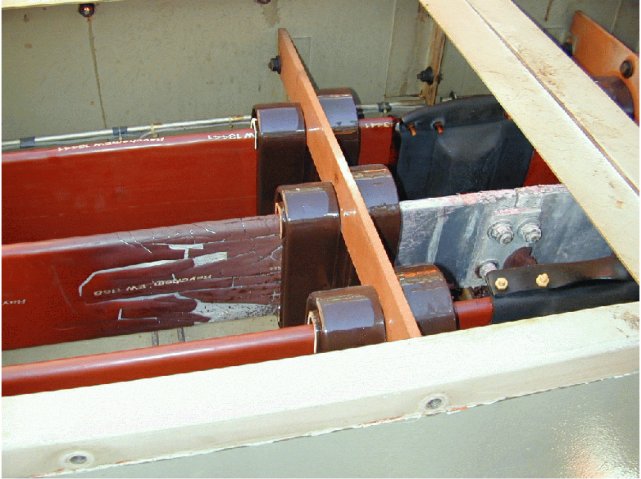
View 2 of BUS 309 Showing degraded Insulation on Bus Bar
