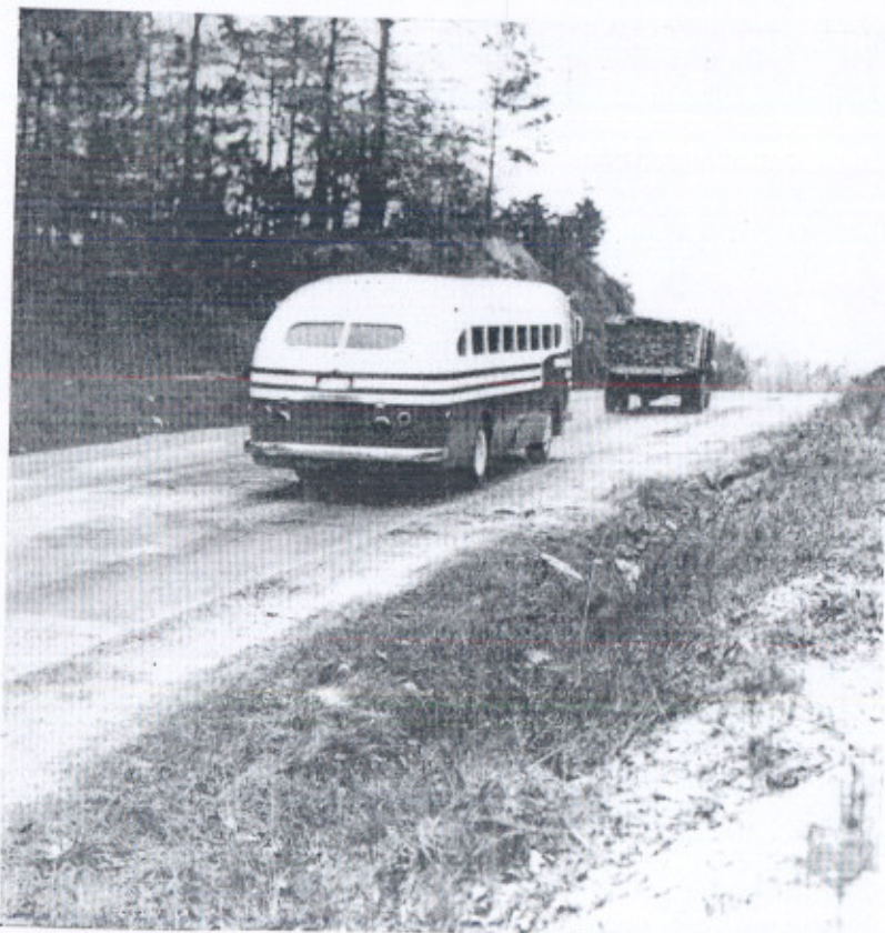
"They shall not pass" at this point on U S Route 78 in Alabama, where sight distance is practically zero. The 20-foot pavement is badly damaged and the shoulders worn and narrow, yet this road must handle 3,350 vehicles daily. Reconstruction to remedy such conditions is required on 14,283 miles of the interstate system.
