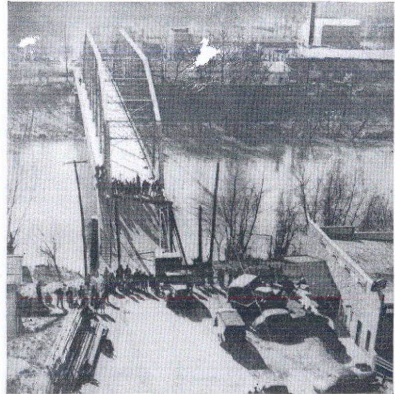
Seriously inadequate in load-carrying capacity are 677 bridges on the interstate system. This one on U S Route 25 in Kentucky, old and too narrow, had one span completely wrecked when an Army truck hit the end post. Some 8,234 bridges on the system fail to meet the interstate standards for load capacity.
