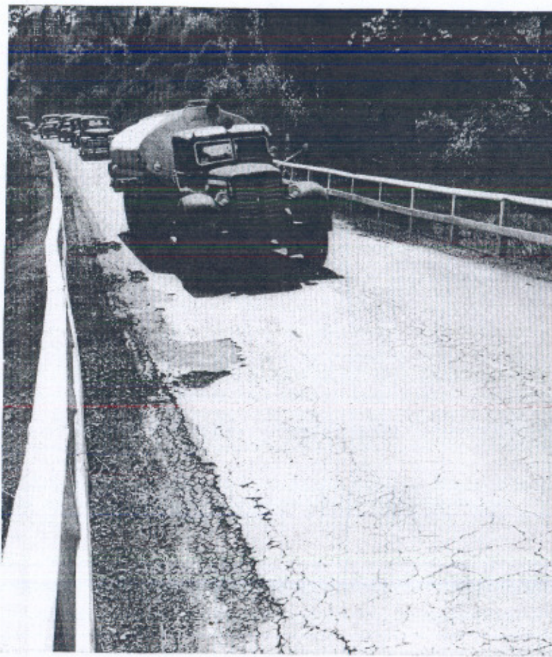
Lines of crawling traffic on hills are not unexpected when the badly broken pavement is so closely hemmed in by guardrails and there is neither passing sight distance nor room to pass. This part of U S Route 40 in California is traveled daily by 4,000 vehicles. Passing sight distance is undesirably restricted on 7,324 miles of the interstate system.
