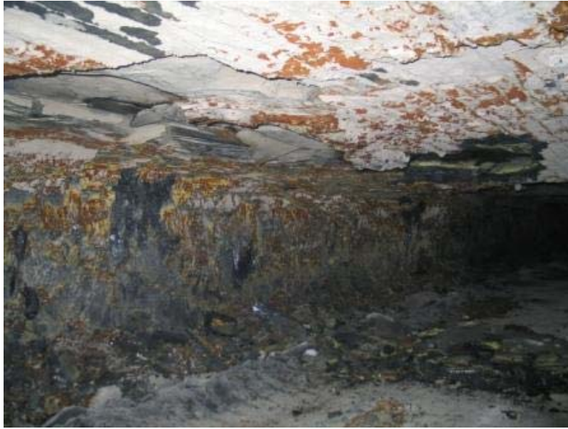
Figure 2.3 A view of the rib and roof condition at the test site of the Nolo Mine.
