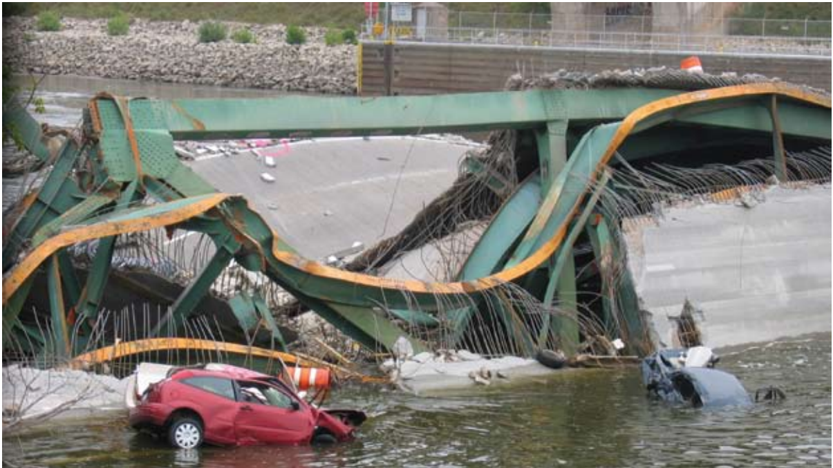
Cars and roadway litter the river where the I-35 bridge collapsed in Minneapolis on August, 5, 2007. (Photo by Todd Swain/FEMA)
