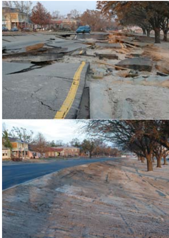
Biloxi, Miss., September 3 and November 3, 2005—U.S. Highway 90 before (top) and after repair from damage caused by Hurricane Katrina. (Photo by Mark Wolfe/FEMA)
