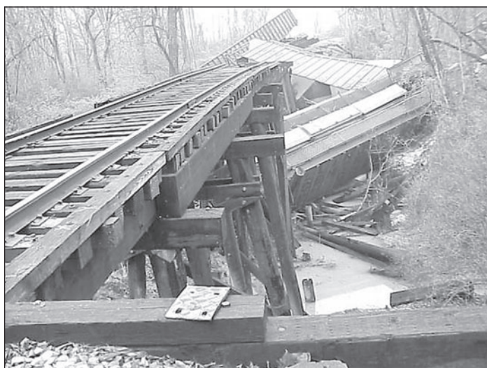
Figure 5: Structural Failure of a Bridge in Mississippi
