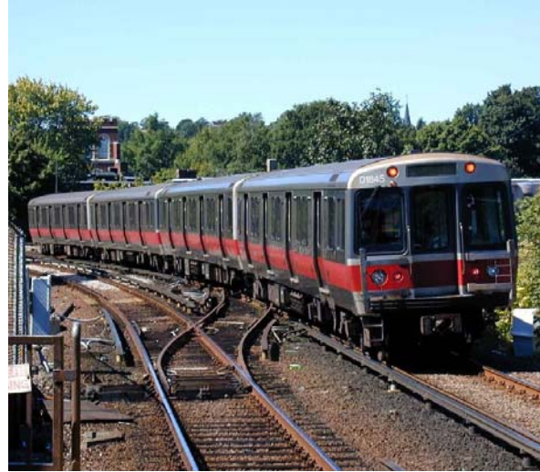
Switch and signal equipment provide essential functions for a rail line.
