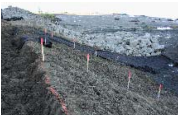
Construction sequence showing the completed slope, key trench, geotextile, and rock riprap
