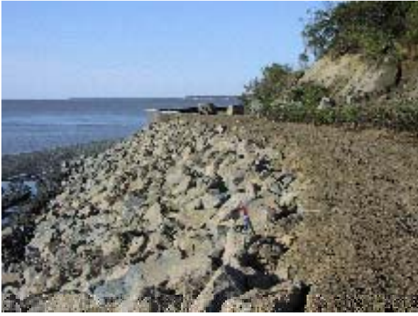
Completed riprap slope protection. The disturbed area was seeded and willows were planted.
