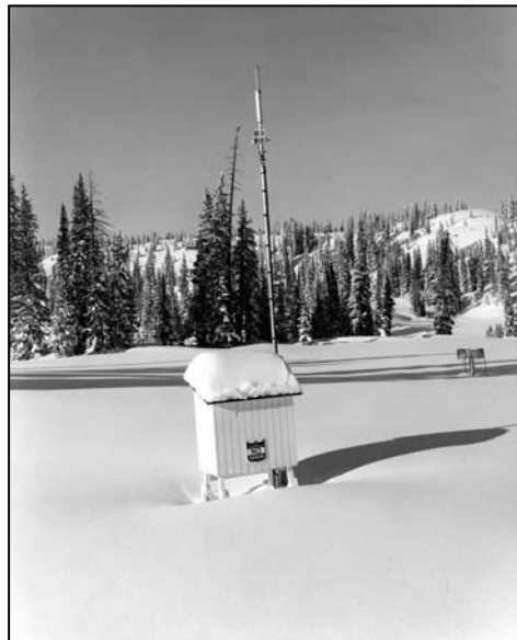
4.22 Repeater at Park Range transmits data to base station at Steamboat Springs, Colorado
