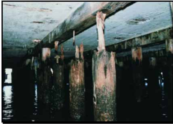
Figure 1. Photo. Marine borers ( Limnoria ) attacking untreated timber piles that support many of New York's highways and harbor piers. (9)
