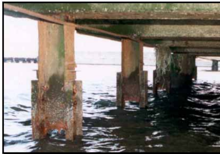
Figure 2. Photo. Complete corrosion of steel H piles supporting a harbor pier (recently installed retrofit channels are already corroding). (9)
