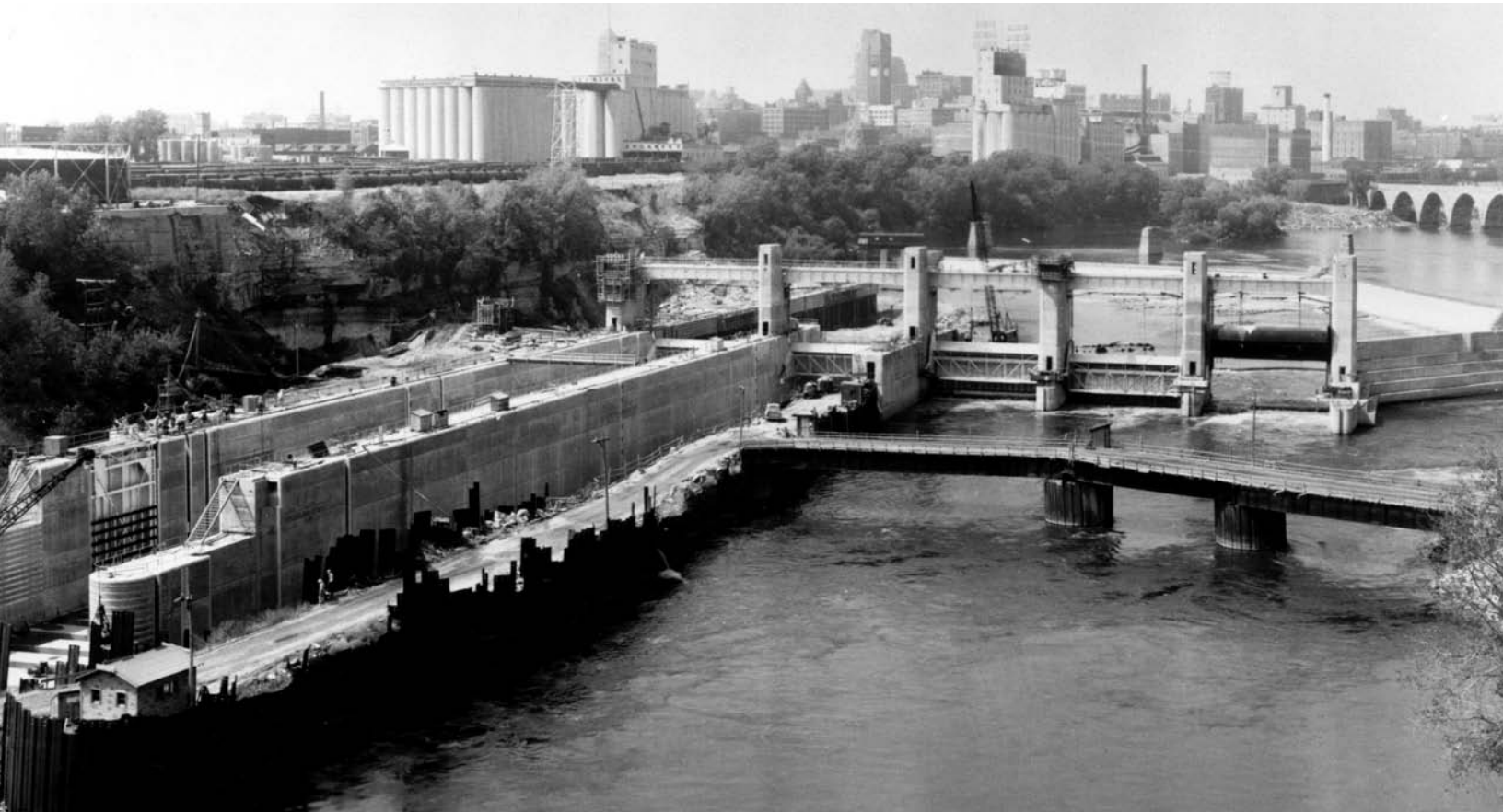
FIGURE 9. Lower St. Anthony Falls Lock and Dam under construction, 1956. St. Paul District, Corps of Engineers.
