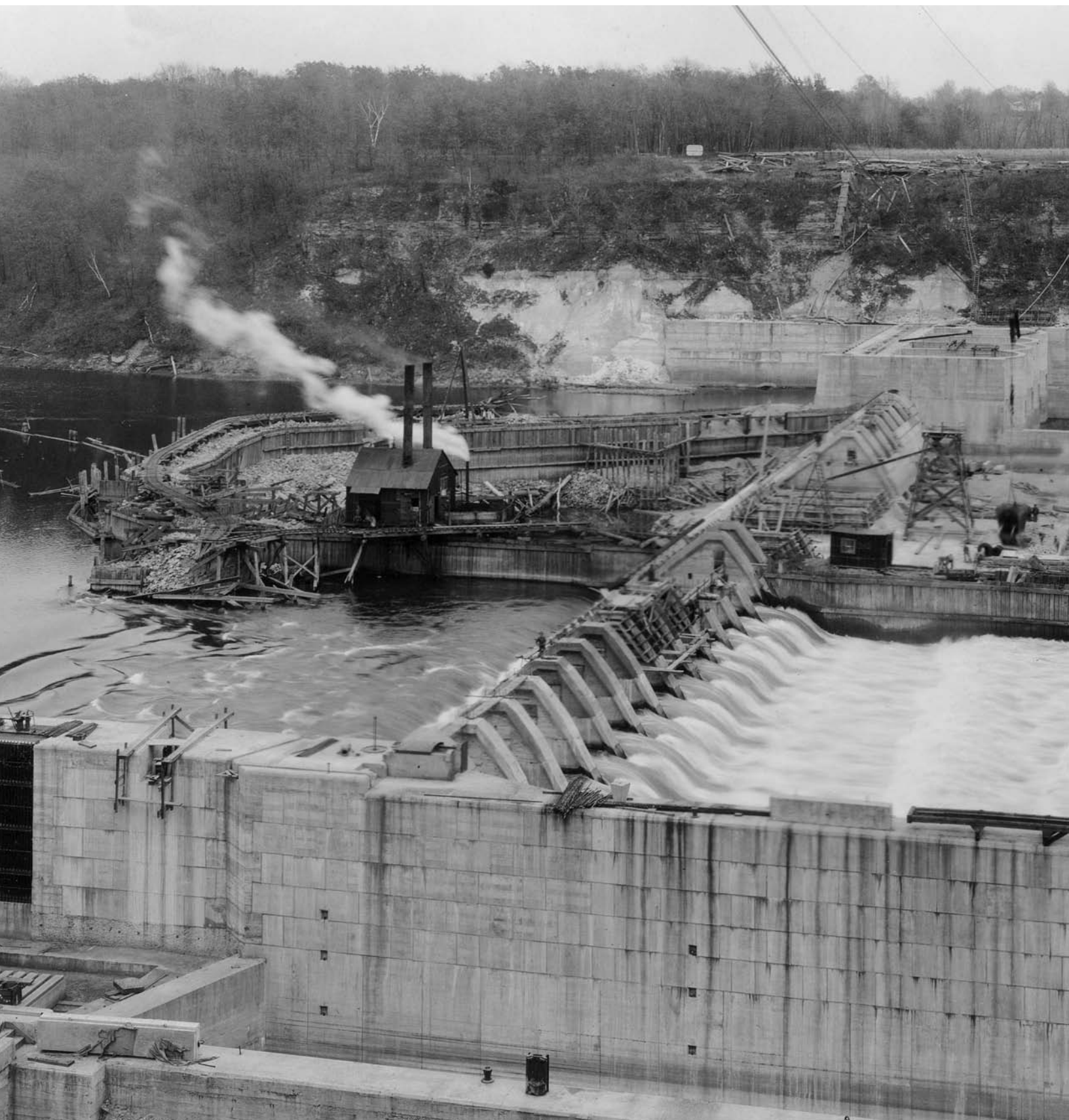
FIGURE 1. Lock and Dam No. 1 under construction, 1916. St. Paul District, Corps of Engineers.
