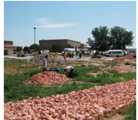
TANF Summer Youth Corps work on a water conservation focused landscaping project for Weld County Government
