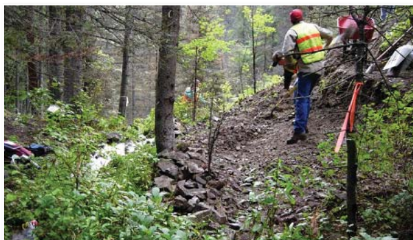
Waste rock being removed from the area below a newly constructed recreational path in Red River, New Mexico.
