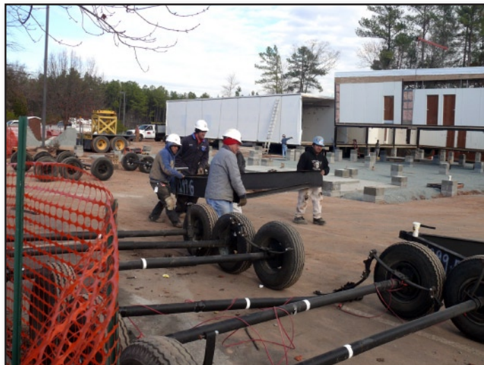
A portion of the main road through campus was closed as the modules were trucked in. (Photo courtesy of Steve McCaw and John Maruca)
