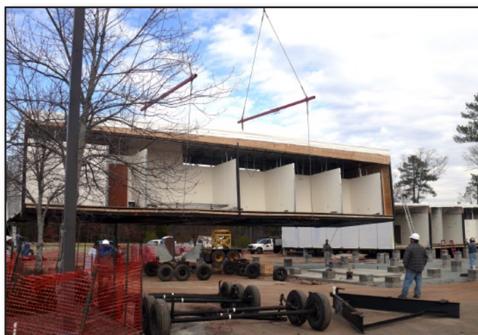
One by one, workers guided the units into place as the larger structure emerged. The units, which measure 15 feet by 77 feet, contain the wiring, walls, insulation, windows and even the office doors and door locks. (Photo courtesy of Steve McCaw and John Maruca)
