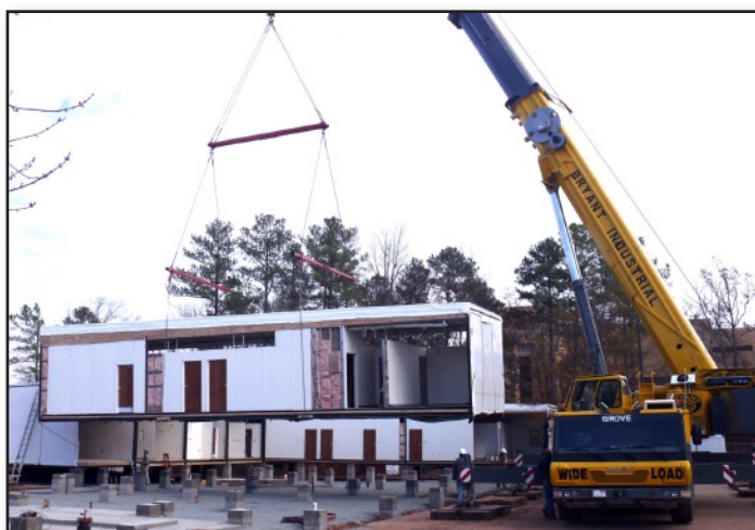
A powerful crane lifted the units into place. The modules were pre-constructed in Pembroke, NC, fitted together and then taken apart before being trucked to the site. (Photo courtesy of Steve McCaw and John Maruca)
