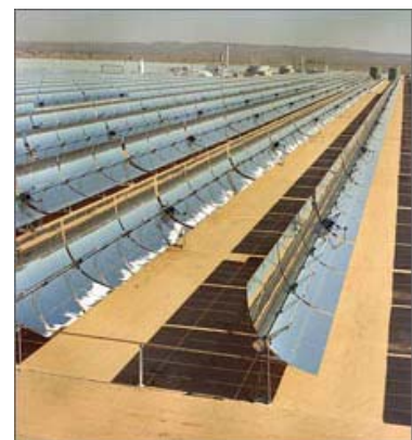
Fig. 2. Array of parabolic troughs at the Kramer Junction Solar Concentrating Plant.
