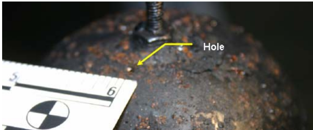
Figure S- 6. Close-up of LSH-5020 float, showing corrosion and hole
