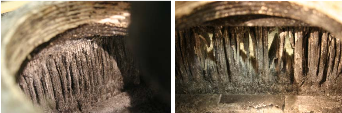
Figure 10. Flame arrester plate corrosion (inside)
