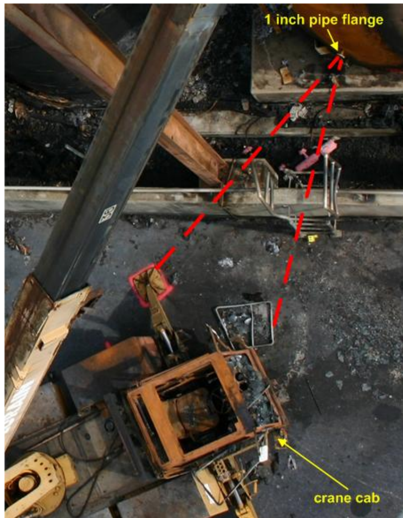
Figure 6. Methanol spray from 1-inch pipe flanges onto the crane cab.
