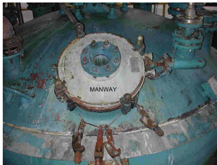
Figure 6. The 18-inch reactor manway.
