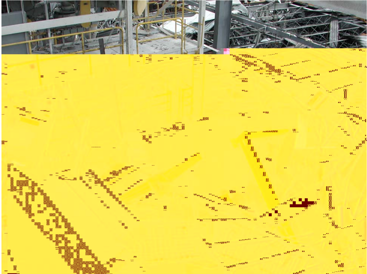
Figure B-2. Area between mixers #1 and 2. (Note upward heave of broken concrete floor.)
