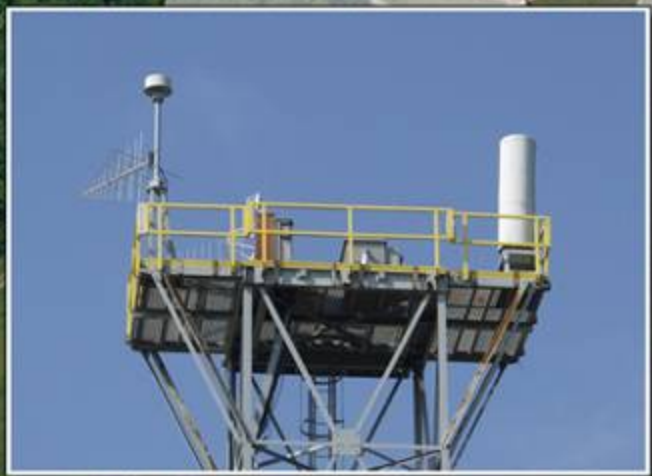
UHF Command Receive & Frequency Monitoring
