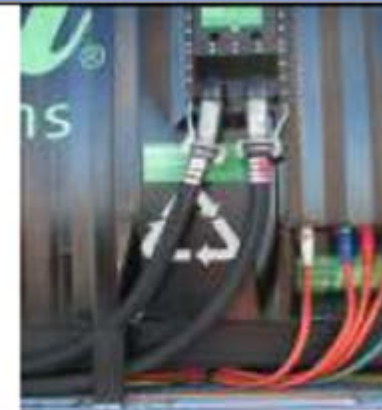
Data Power Cooling
