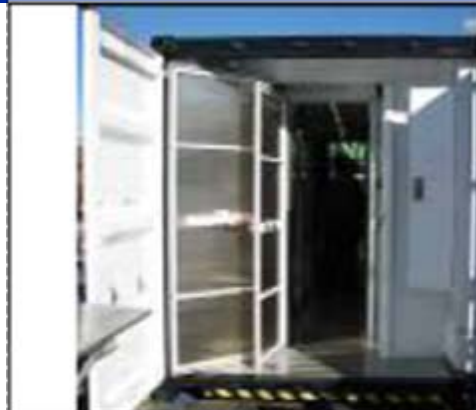
7 Racks plus Network
