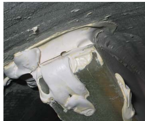
Figure 25: Crack at shear web termination on the LP surface of the BSDS blade.
