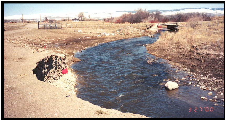
Figure 1: Eroding bank on the Jack Webster Ranch, lower end of Medicine Lodge Creek about 15 miles West of Dubois, ID in March, 2000.
