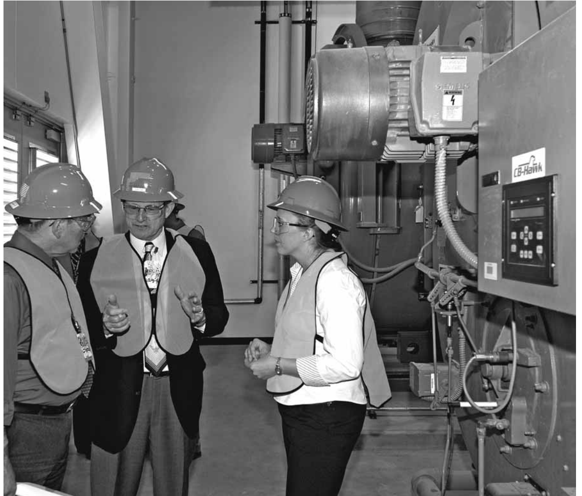
ES&H WALKTHROUGH — Sandia Director Tom Hunter, center, talks about Environmental, Safety, and Health (ES&H) issues with Sam Varnado, director of Center 12100, and Joanna Eckstein (10333) during a recent walkthrough of the MESA Central Utility Building (CUB). Joanna is part of Sandia’s air quality division and was assisting during the walkthrough. (Photo by Bill Doty)
