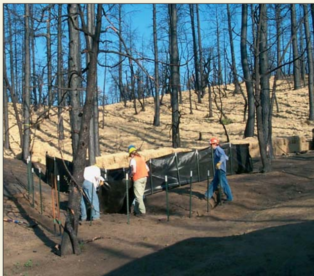
Installation of silt fences at the mouth of a treated catchment on the Indian Fire mulch treatment study on the Prescott National Forest.
